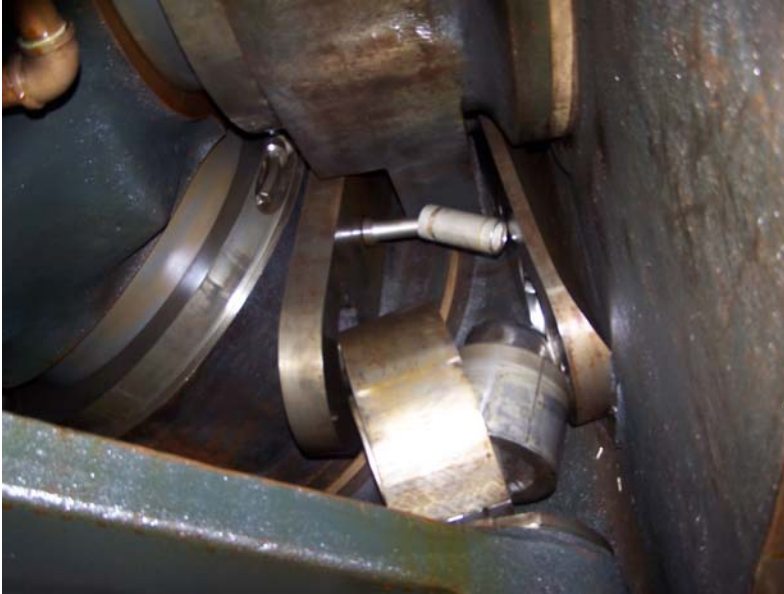
Photo A-4. Inside of the Runner Hub Showing Broken Linkage, John Day Unit 16
